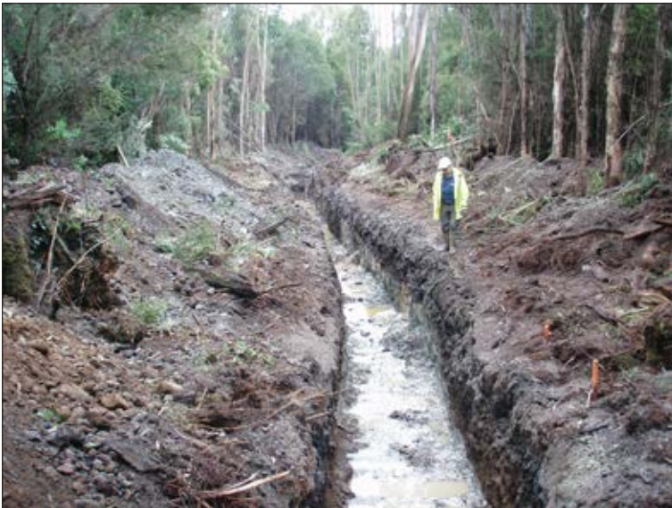
Costean at Stanley Reward showing topsoil to right and gravel to left.
