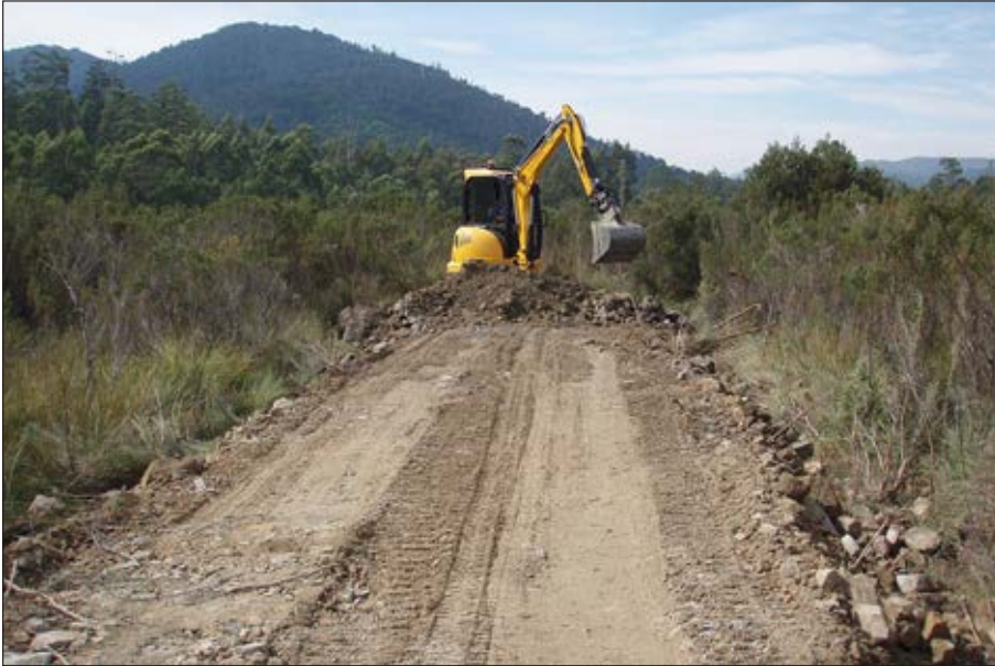
Track construction through buttongrass on peat — coarse fill from local borrow pit.
