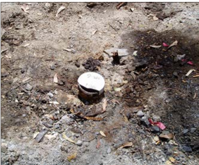
Broken PVC cap on steel collar.
