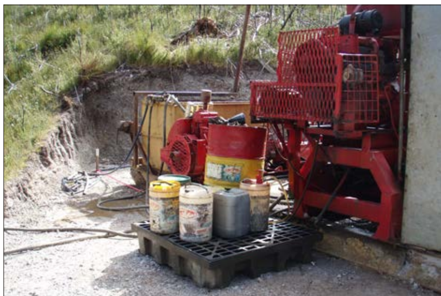
Bunded hydrocarbon storage — but no tarp or roof cover.
