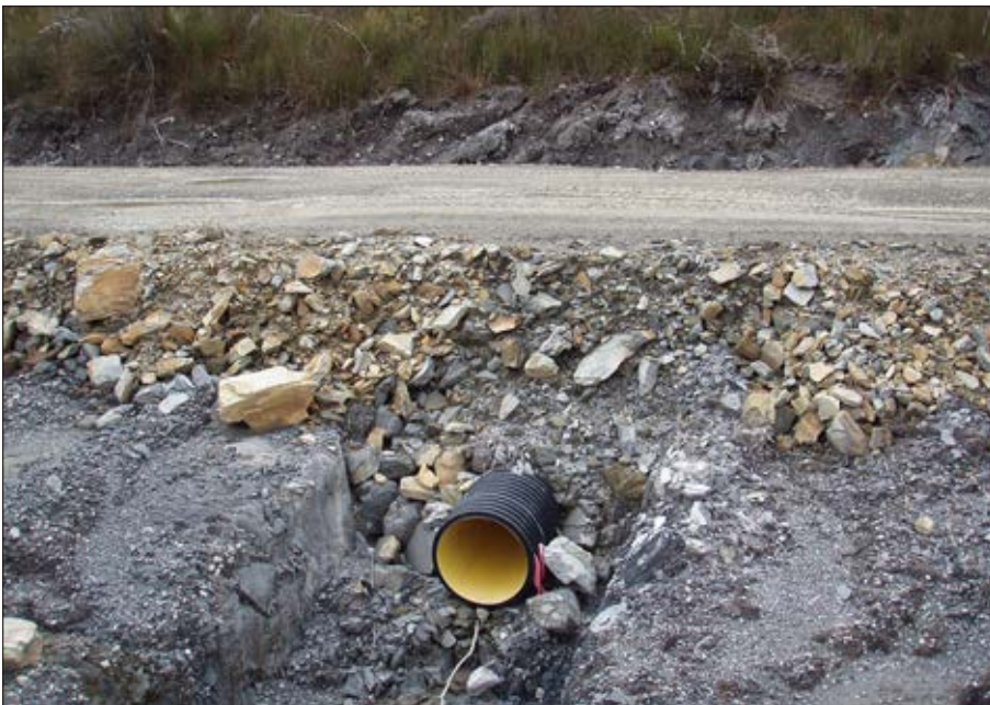
Note rip rap in discharge area and good foundation.
